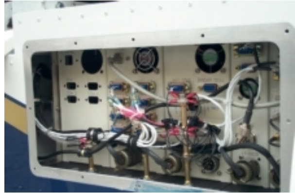
Figure 3 – Wiring on “back” side of module rack, note that in this particular picture computer module #2 on the left is empty
