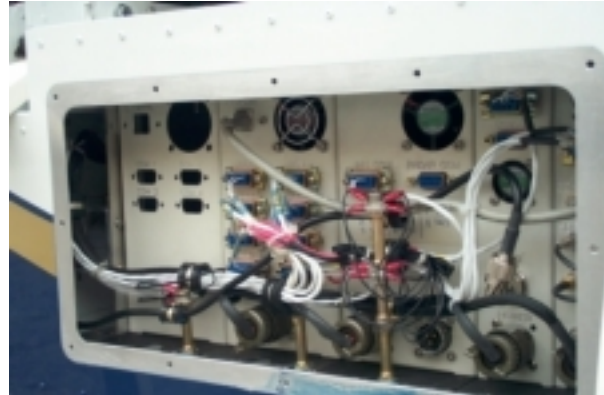
Figure 3 – Wiring on One Side of Module Rack
